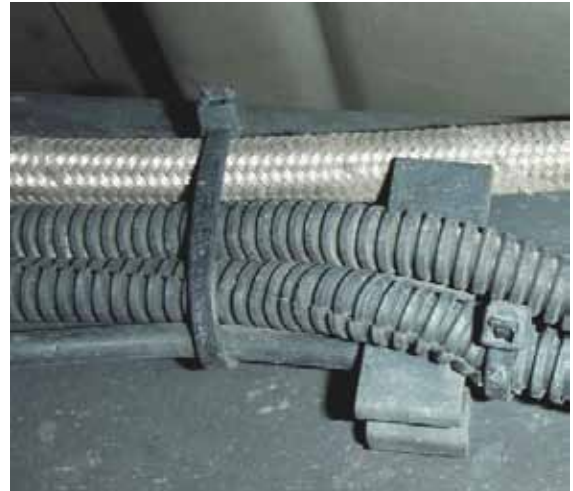
Figure 54. Fuel line secured in original location by plastic zip-tie
