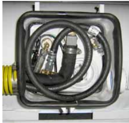
Figure 35. Hoses and vent line in vapor seal box after removing the cover shown in Figure 33.
