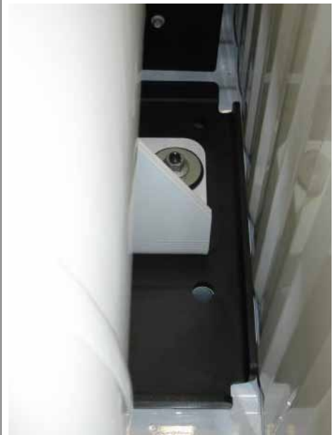
Figure 23. OEM engineered tank-mounting installation
