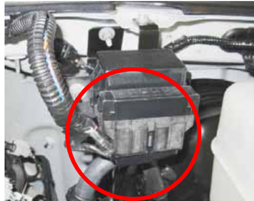
Figure 63. Relay control panel
