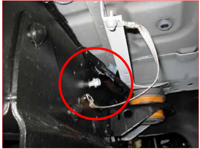
Figure 48. Disconnected ground strap
