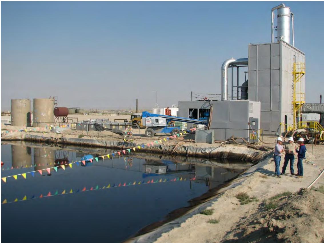
Figure 10. Treatment facility at the Jonah Gas Field, Sublette County, Wyoming used to separate condensate, methanol, brine, and water from drilling fluids. (USFWS Photo by P. Ramirez)
