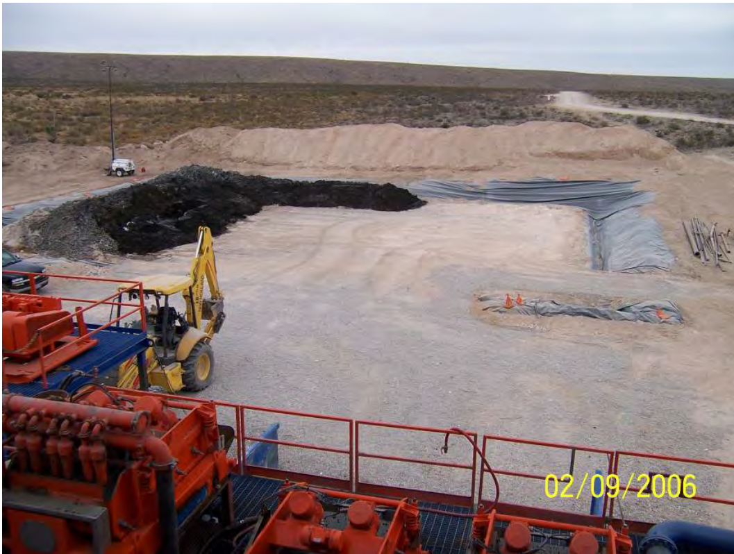
Figure 7. Closed-loop or pitless drilling site with synthetically-lined pad for temporary storage of drill cuttings.
