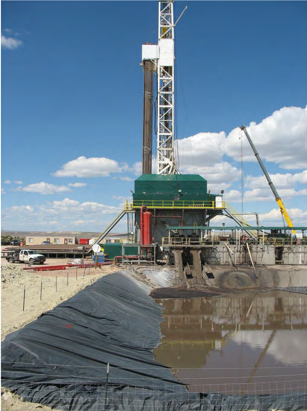
Figure 1. Reserve pit adjacent to a drilling rig near La Barge, Wyoming. (USFWS Photo by P. Ramirez)
