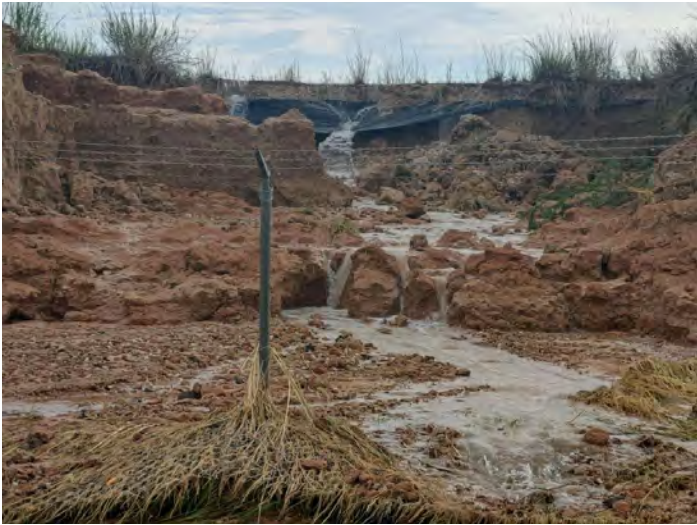
DEWITT COUNTY, Texas - Over 60,000 gallons of rainwater spilled across Hohn Road near Nordheim.
