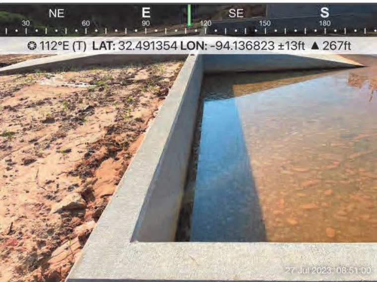
Fluids inside the new unpermitted pit appears to be saltwater.
