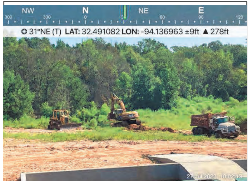
McBride operators are working on the saltwater spill path.
