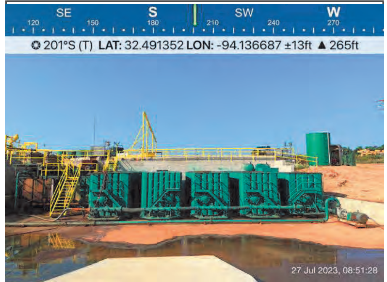
North view of the new unpermitted pit.
